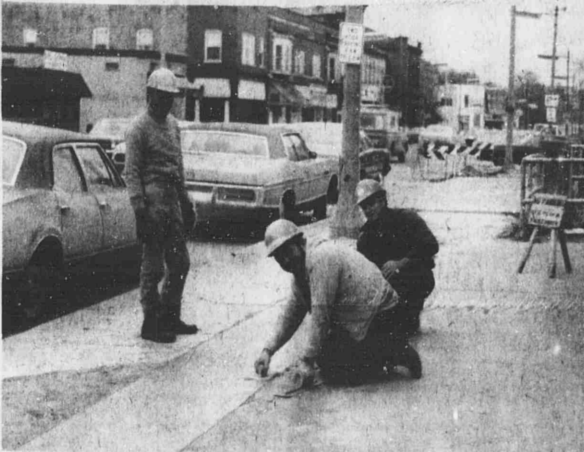
Workmen create a path of new concrete in the repair of torn-up sections of sidewalk resulting from the laying of underground cable by Michigan Bell Telephone Co.
