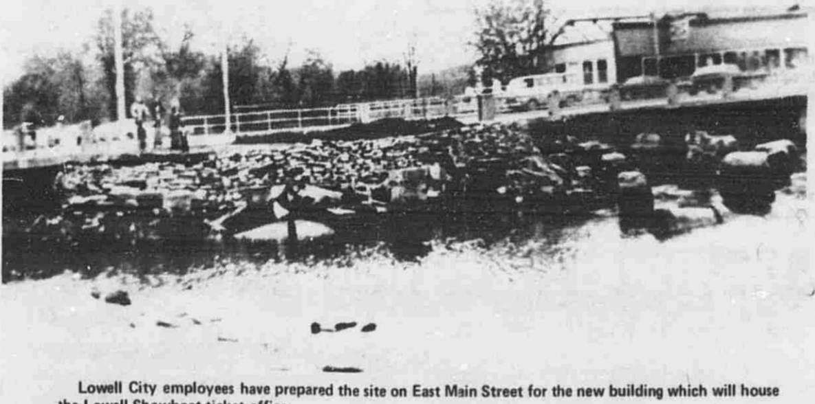
Lowell City employees have prepared the site on East Main Street for the new building which will house the Lowell Showboat ticket office.
