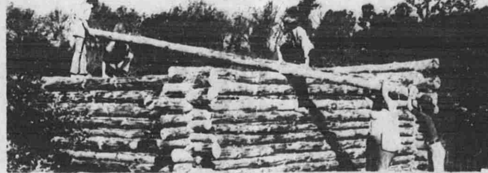
This remarkable log cabin, constructed without nails, is actually being erected behind Lowell Middle School by sixth, seventh and eighth grade students under the supervision of Science Teacher George Stegmier.
