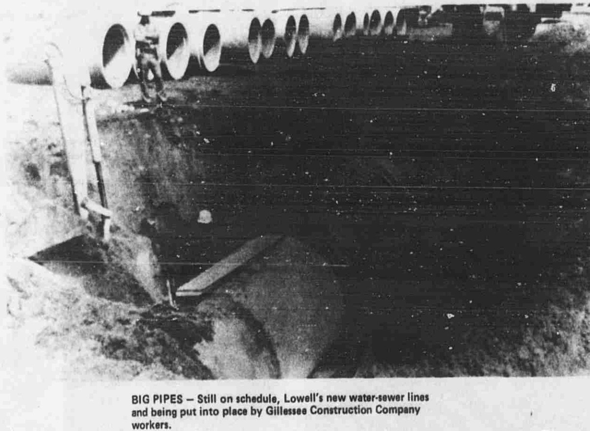
BIG PIPES - Still on schedule, Lowell's new water-sewer lines and being put into place by Gillesse Construction Company workers.
