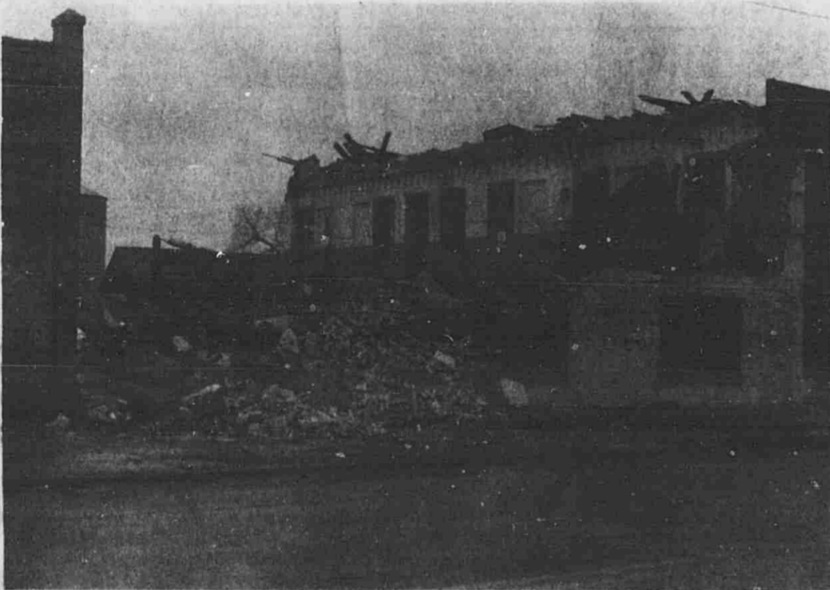
Slowly disappearing, due to the work of a demolition crew, is the former Root-Lowell Manufacturing building on West Main Street.
