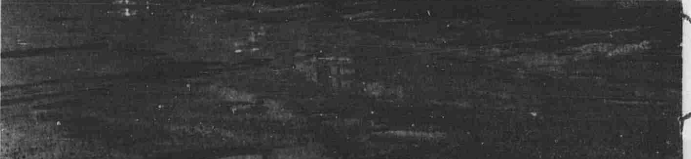
Chuck holes in the city's west side parking lot shows what winter can do to pavement.
