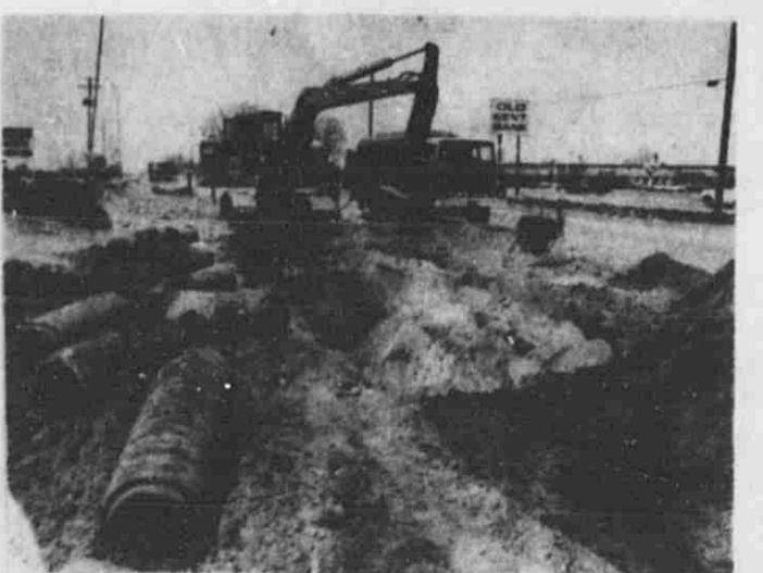
The long arms of the pipe lines which had been steadily inching their public way toward the Village of Cascade, have almost reached their destination. Digging and laying of the pipe for both sewer and water held traffic at bay from time to time as it added to the dust layers in the area, but residents will soon find relief as the final stretch down the hill on 28th Street reaches bottom and total connection.
