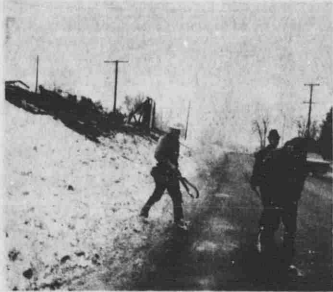
CONSUMERS POWER COMPANY MEN REPAIR LINES DOWNED BY THE FIRE.
