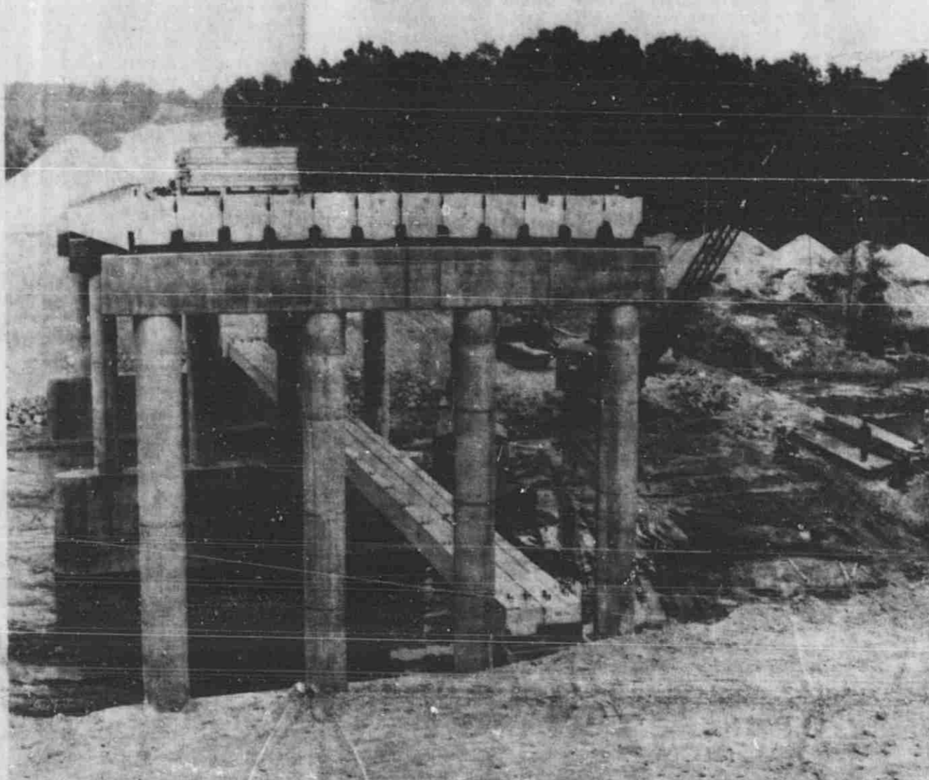
NEW BRIDGE RISING - This is the new Fallasburg bridge rising over the Flat River north of Lowell. It will be part of a highway system carrying east-west traffic between Grand Rapids and Ionia County.
