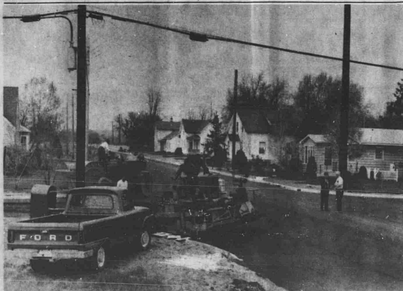
FINISHING TOUCHES — Workmen are shown here completing the job of paving the new Hudson Street extension which links Hudson and Lincoln Lake in Lowell. Now opened to traffic, the new interceptor is designed to produce a smooth flow of north-south traffic through the city.
